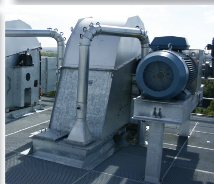
Elevators with discharge suction intakes
