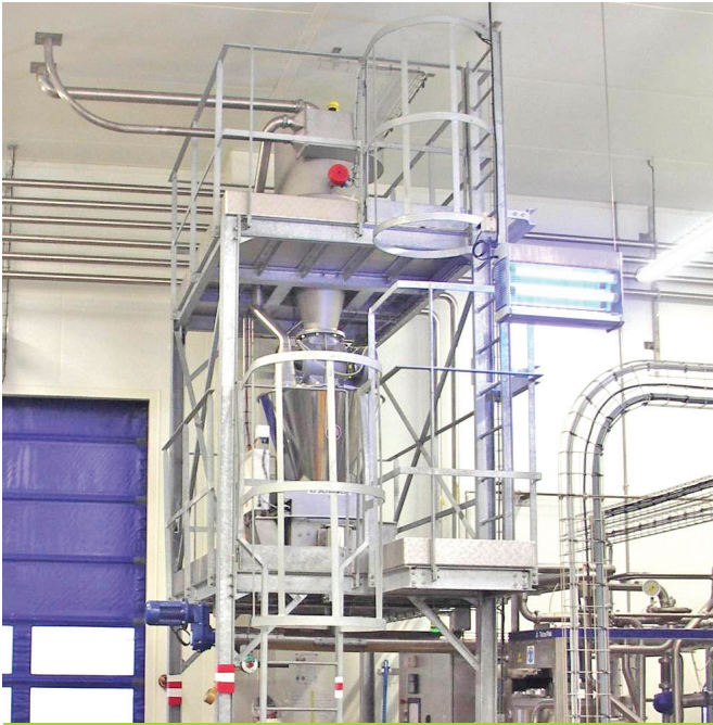
A pneumatic transfer supply by cyclone
