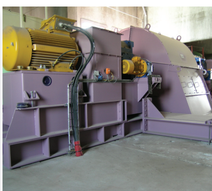
High capacity elevator head (1600 m 3 /h, height 65 m, 2x200 kW)
