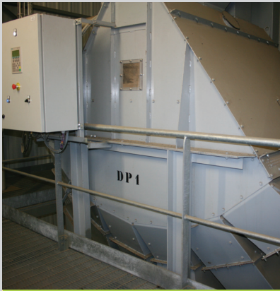
Swing spout distributor and control cabinet
