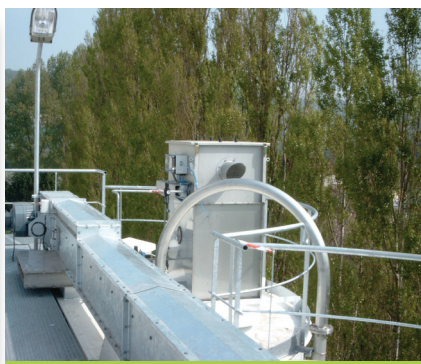
Pads filter for silo depressurization
